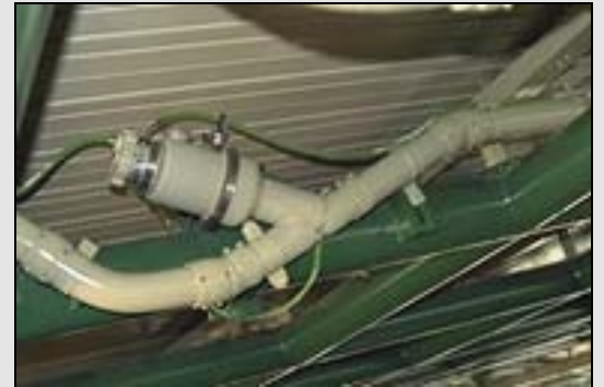
Iseki Vacuum Interface valve suspended in roof
