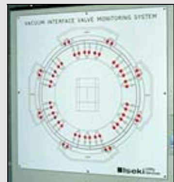
Valve monitoring panel located in pump station
