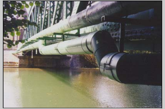
Vacuum sewer main crossing the river
